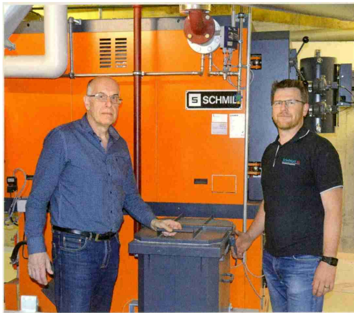
Bilder: Schmid Energy Solutions
